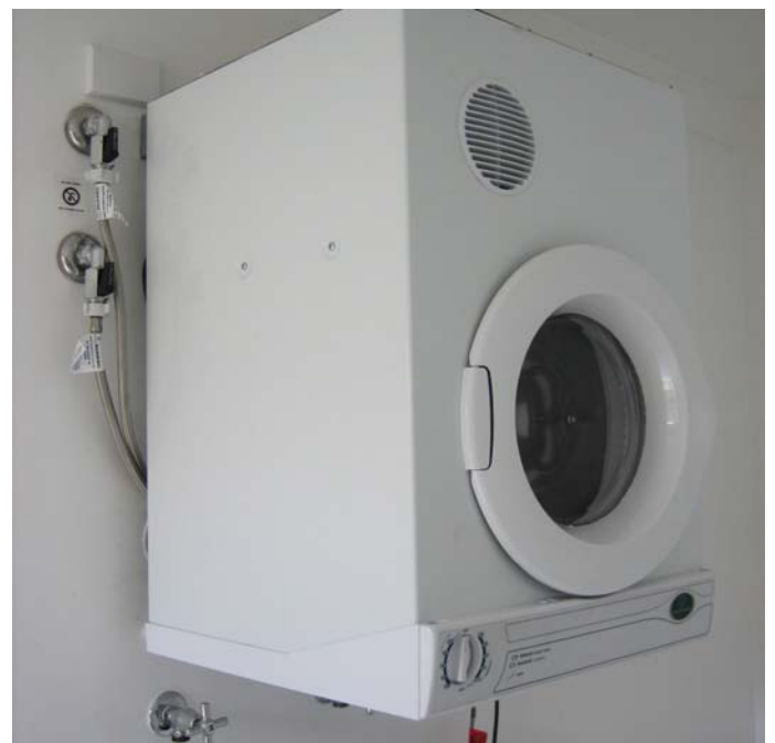
GridX generating waste heat is used in home appliances, such as this hydronic clothes drier.
