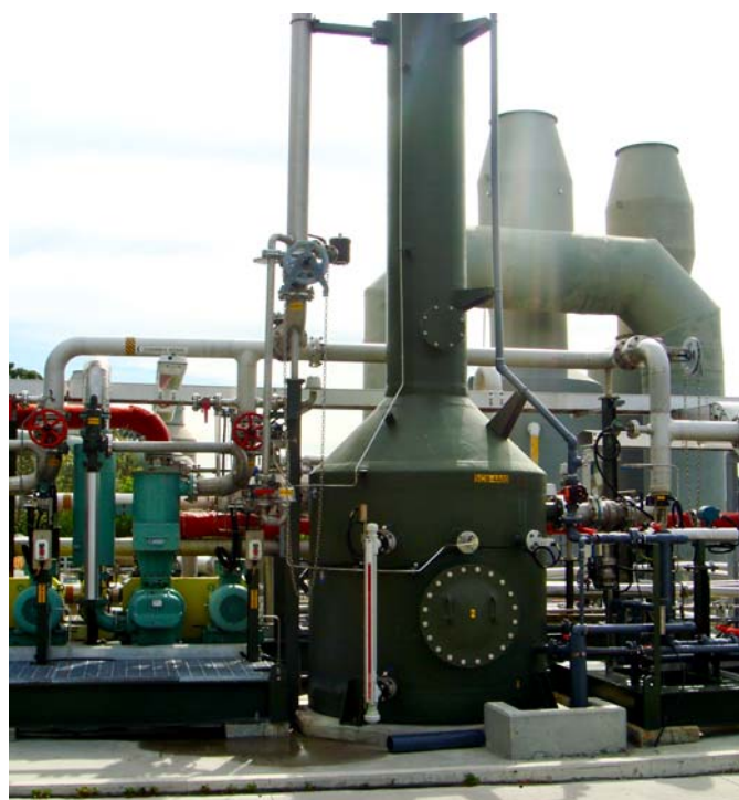
Figure 1: Scrubber system for the sewage gas (biogas)
