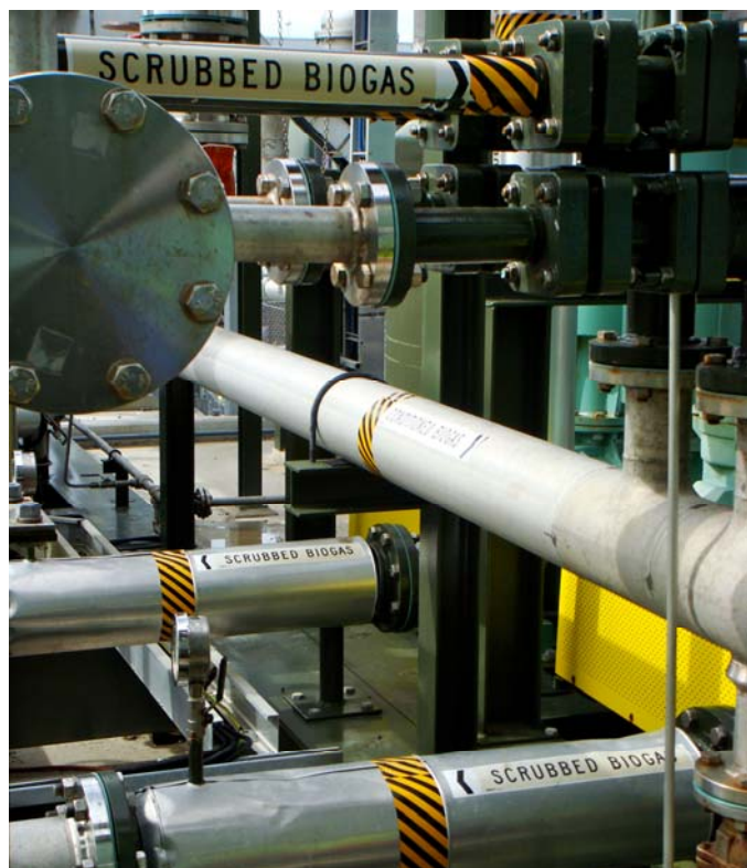
Figure 3: Piping for biogas scrubber system
