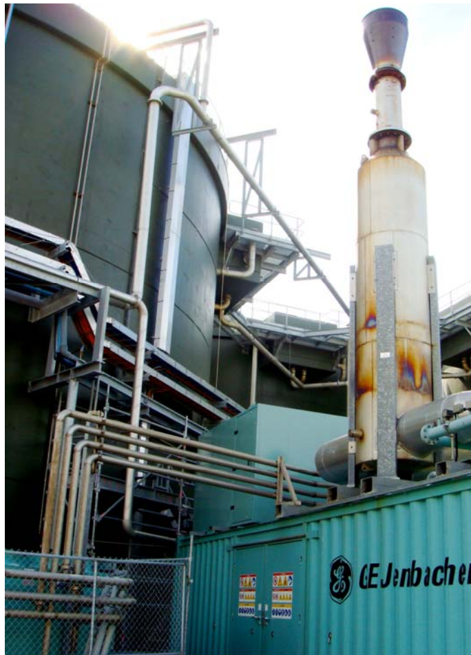
Figure 2: GE Jenbacher cogeneration unit
