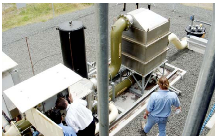
Gas supply connecting to the gas metering system
