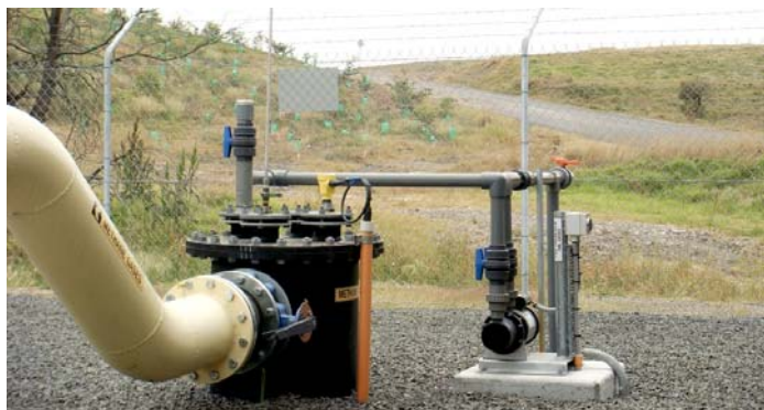
Methane supply from the Grange Avenue landfill
